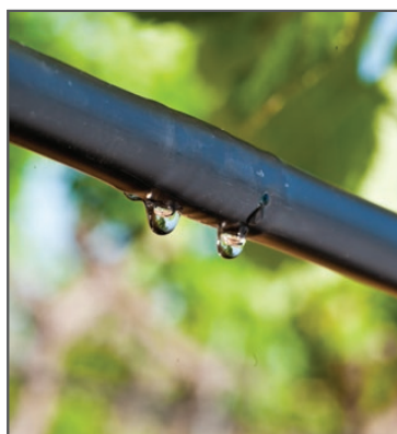
Drip Line Suspended on Wire
